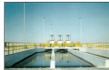
Ismailia Water Treatment Sluice Gates
